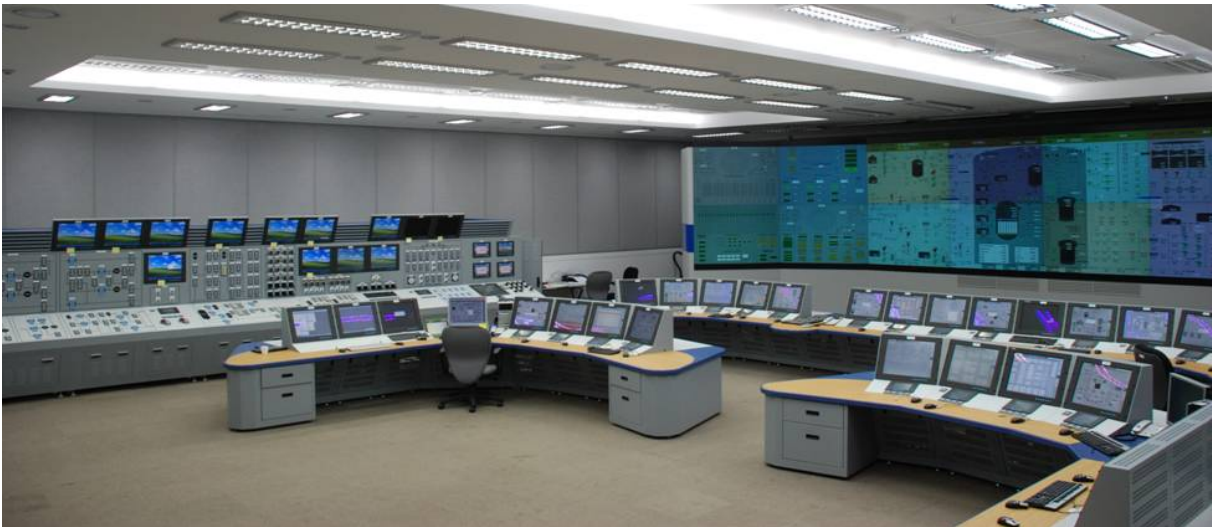
Fig. 1. Main control room's picture of performance test facility
